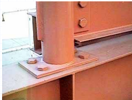
The column delivers a concentrated load to the beam and a bearing stiffener is used on the web
